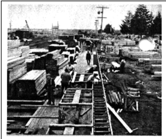
The building of Levittown, NY. A mile of DeWalts (farther than you can see), lumber, roller tables and men. (Photo, 1948)
